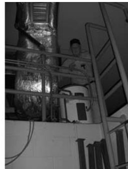
Building and Grounds Committee Chair Everette Tucker surveys various features of the Historical Society's infrastructure that require prompt repair or upgrade.
