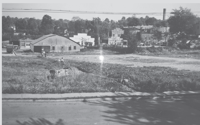
Figure 1. American Legion Property during Installation of Sewer Line Extension in 1949, View (looking east) from Bellevue Avenue (Woman’s Club Scrapbook, n.d.).
